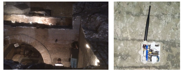
(b) Paper authors installing I/A devices. (c) I/A device in place.
